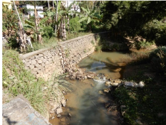
Side protection work in Mangavayal watershed that was partially damaged during the flood of August 2018
