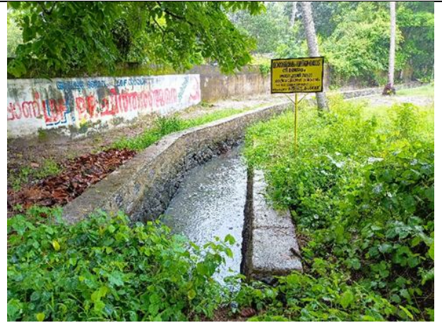
Side protection at Karipozhi
