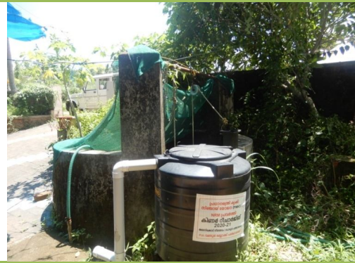
Well recharge structure
