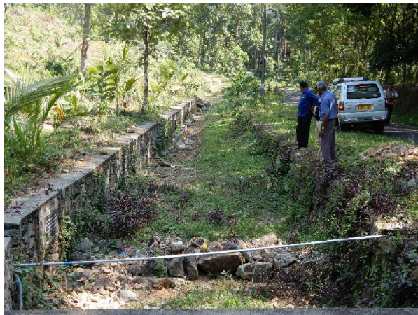
Arukulathod side protection
