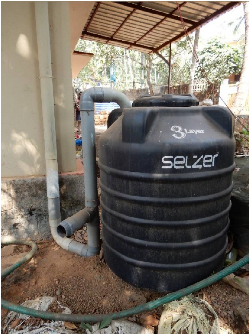
One of the roof top water harvesting well recharge structures installed in Asarithodu watershed
