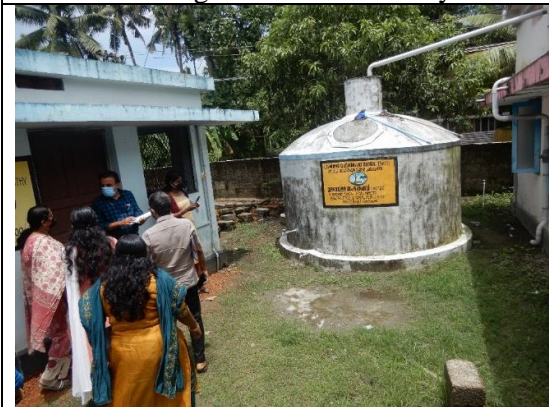
Rainwater harvesting tank at SNGSUP school, Kakkathuruthy watershed
